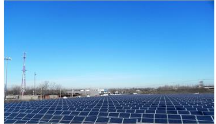
The Cuyahoga Metropolitan Housing's solar field located on the city's east side.
